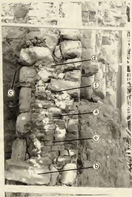
Fig. 17. Cross-section of west wall of nave. The outer and inner face of the wall consists of brick (a), yellow (b) and green sandstone(c), and the core of the wall of rubble stone (d), brick (e) and lime based mortar (f).
